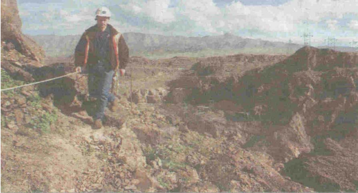
Chris Offe, assistant project manager for the Hoover Dam bypass, walks along the Nevada approach to the Colorado River bridge, due for completion in 2008. It could open northwestern Arizona to development. Photos by Mark Henle/The Arizona Republic
